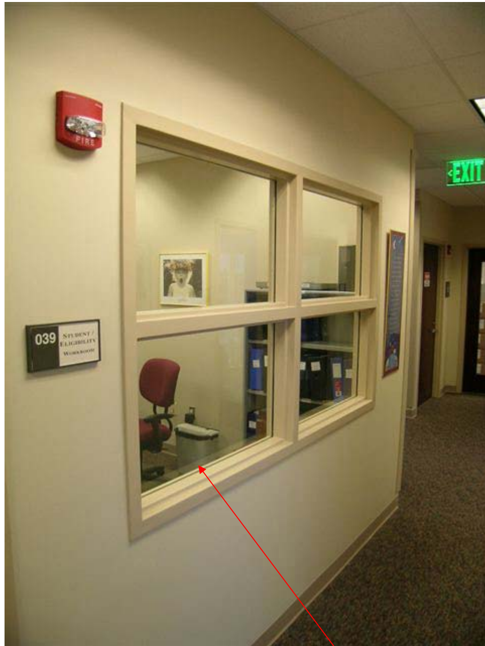
Standard interior view window condition with applied glass stop on “secured” side of frame.
