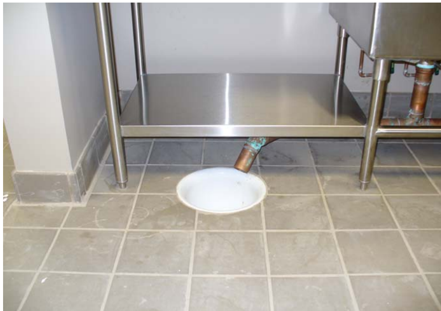
Properly installed floor sink. Drain rim level with adjacent surface.
