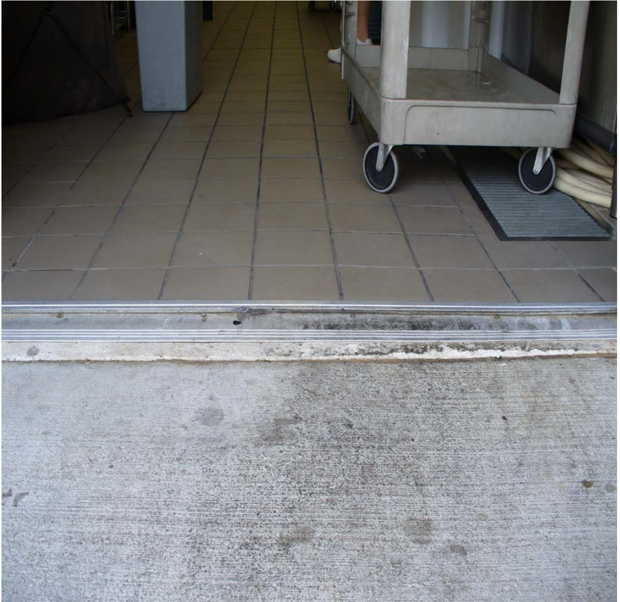
Proper installation of loading dock threshold. Smooth transition and no interferences with hardware.
