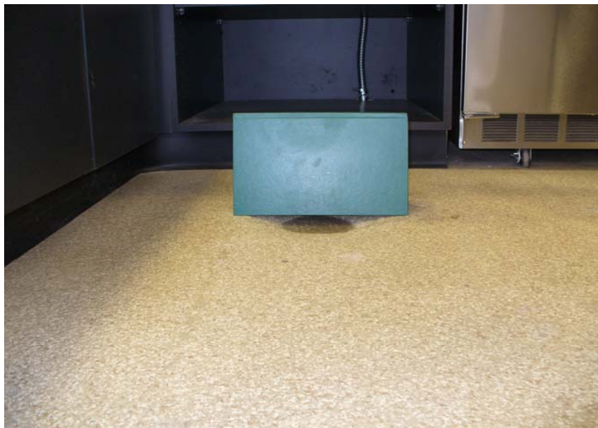
Improper cleanout. Not flush with floor surface.
