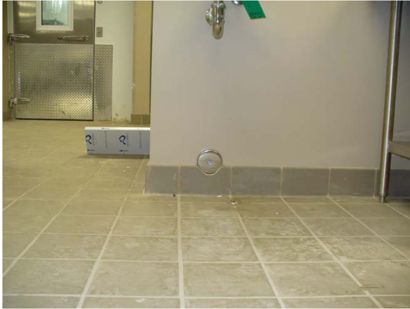
Improper cleanout. Cover should be located above base.
