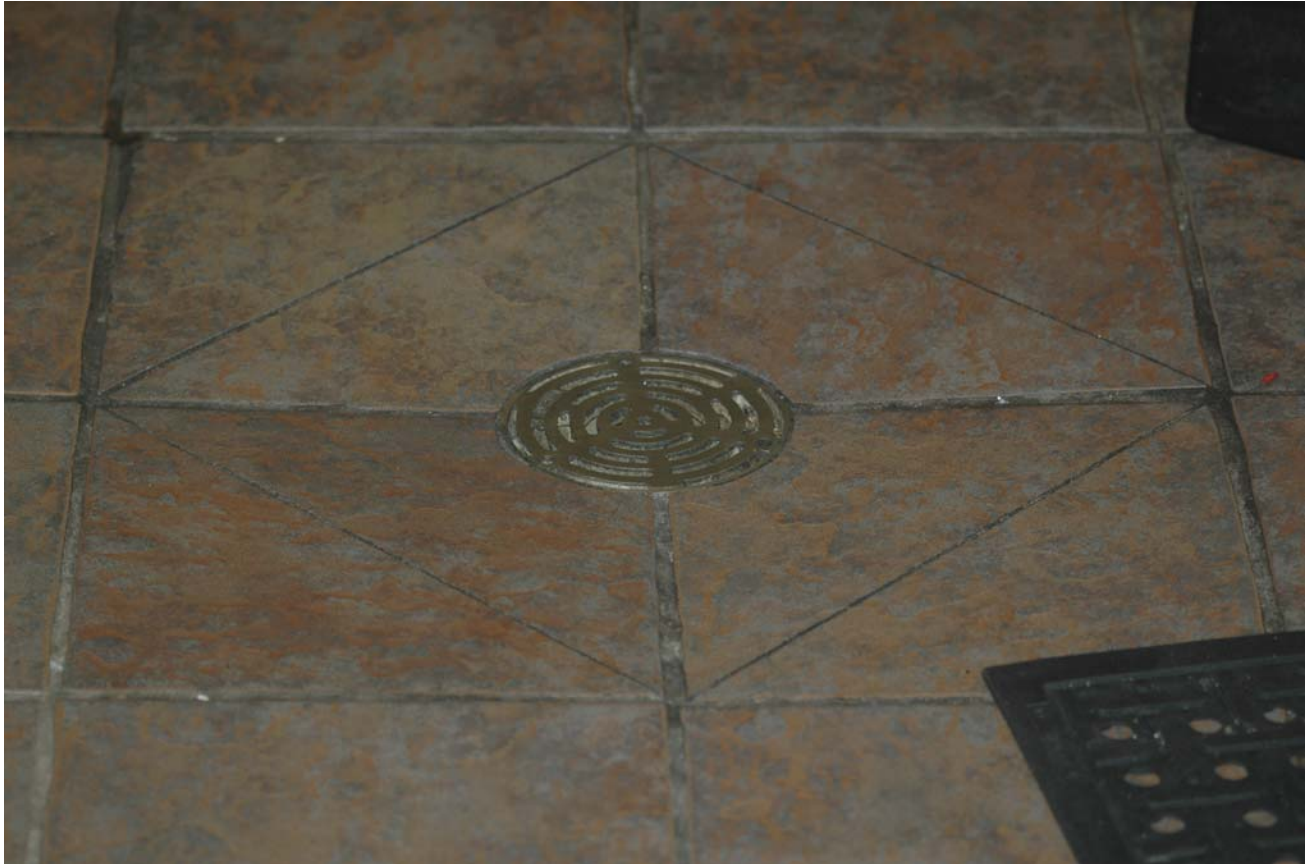
Floor Drain with Proper Slope and Coordinated with Tile Pattern.
