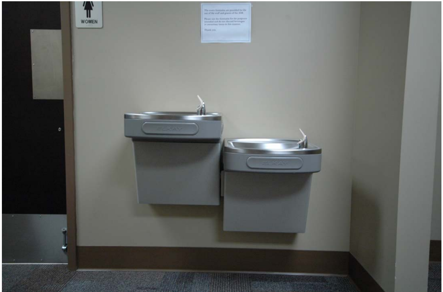
Standard high/low electric water cooler installation
