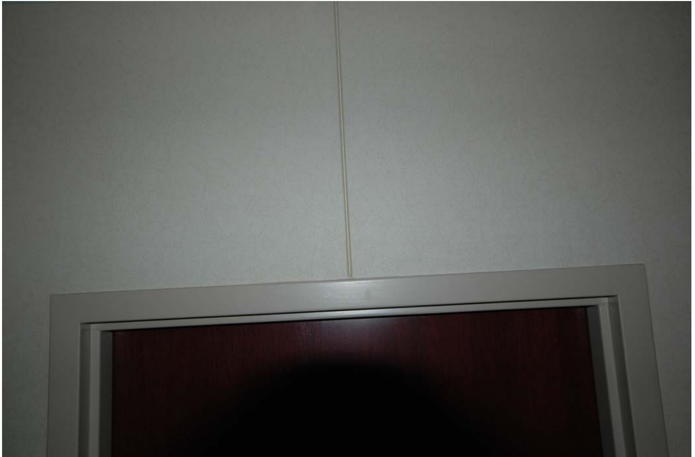
Standard drywall joint installation centered on door frame To be installed and spaced for USGA standards
