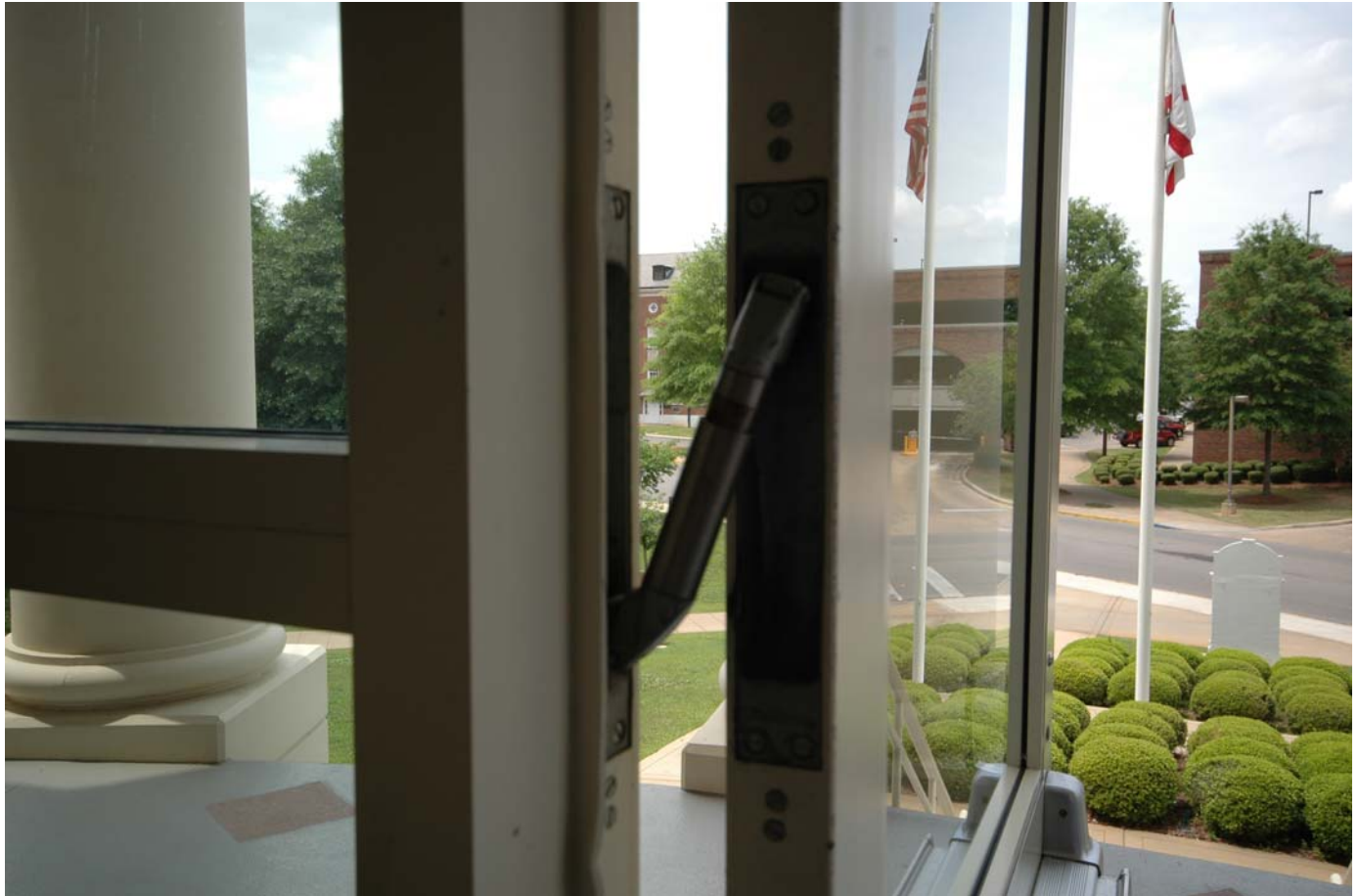
Concealed installation for Electrical Power Transfer (EPT).
