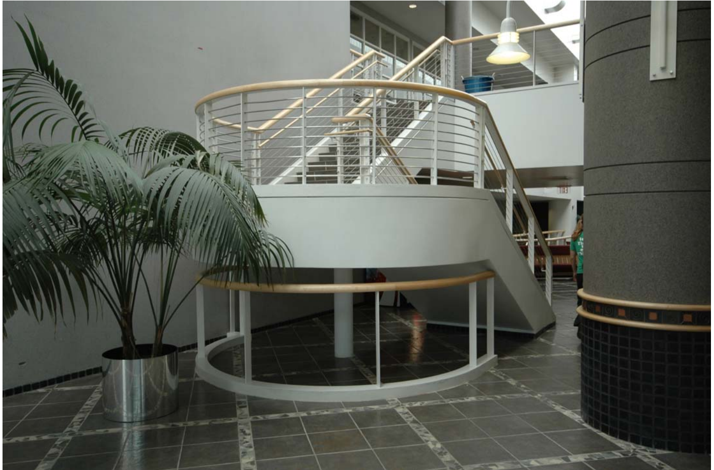
“Cane detection” area installation below stair landing.
