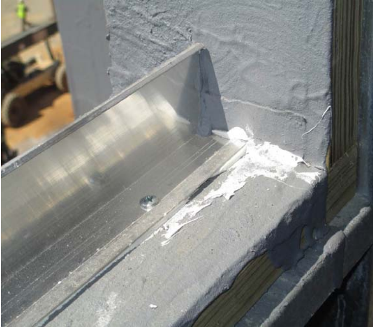
Figure 2: Interior side of a properly installed interior trim angle with liquid membrane flashing pan end dam. Anchor must be cap sealed. Fabric shall not be used.
