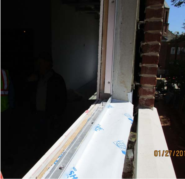
Figure 4: Continuous interior trim angle improperly flashed. No membrane flashing shall be used. LAMF is too thin and not installed to the back of the trim angle. All joints must be sealed water tight. All screws must be cap sealed.
