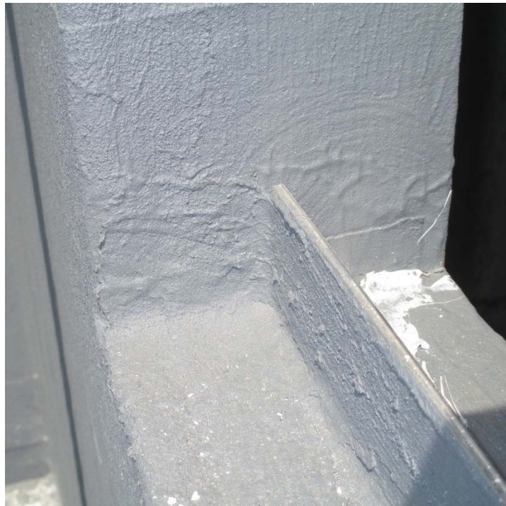
Figure 1: Exterior side of a properly installed interior trim angle with liquid applied membrane flashing pan end and back dams. Fabric shall not be used.
